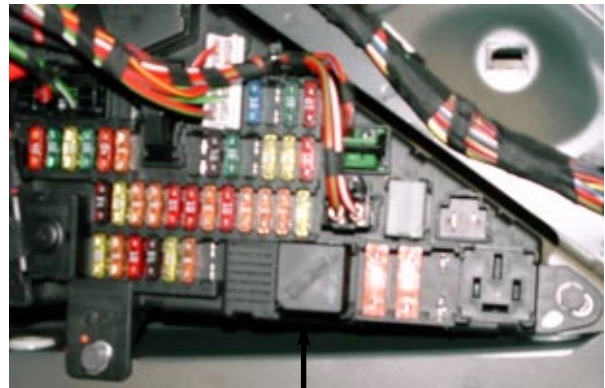
Terminal 30g relay location
